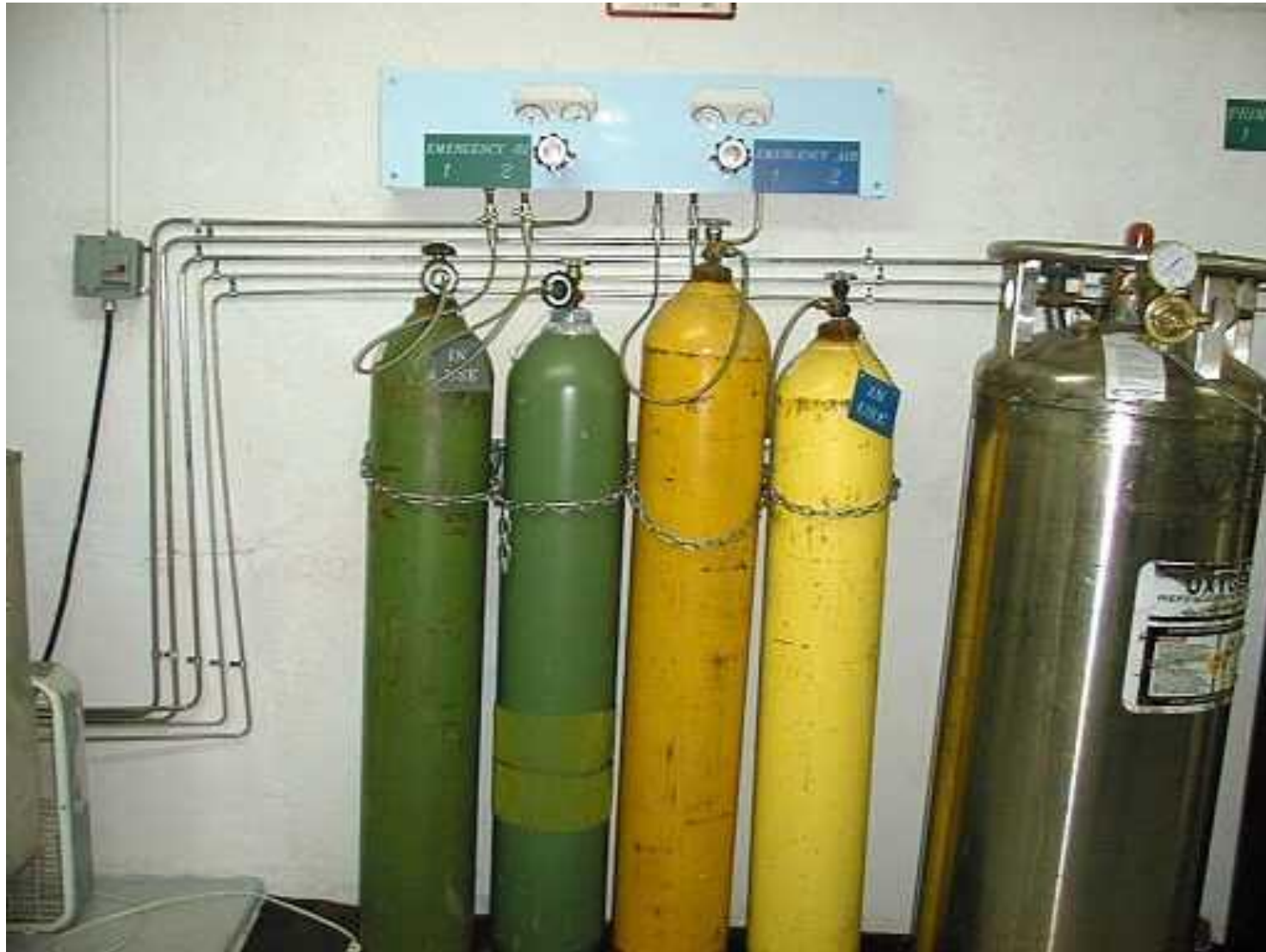
Oxygen Storage (at former location)
